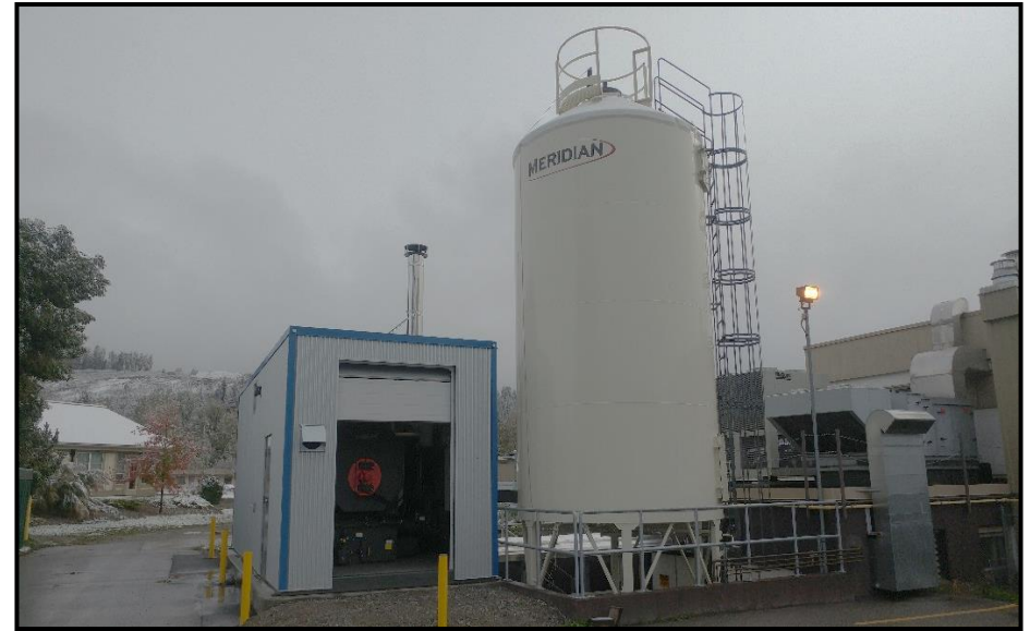
Containerized Biomass Boiler
